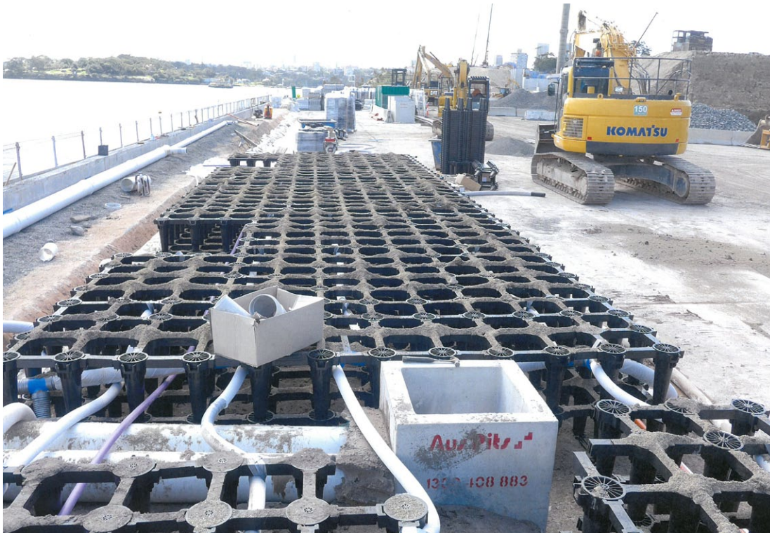
Figure 4.9 – Numerous methods are now available of integrating trees and the necessary soil volumes within urban environments while still allowing pavements and roads to continue successfully above. The above illustrates the proprietary system Strata Vault by Citygreen being used at Barangaroo Sydney.
