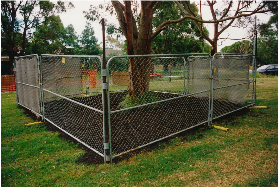
Figure 5.1 – Example of appropriate TPZ mulching, tree protection and construction fencing (Photo: Arterra)
